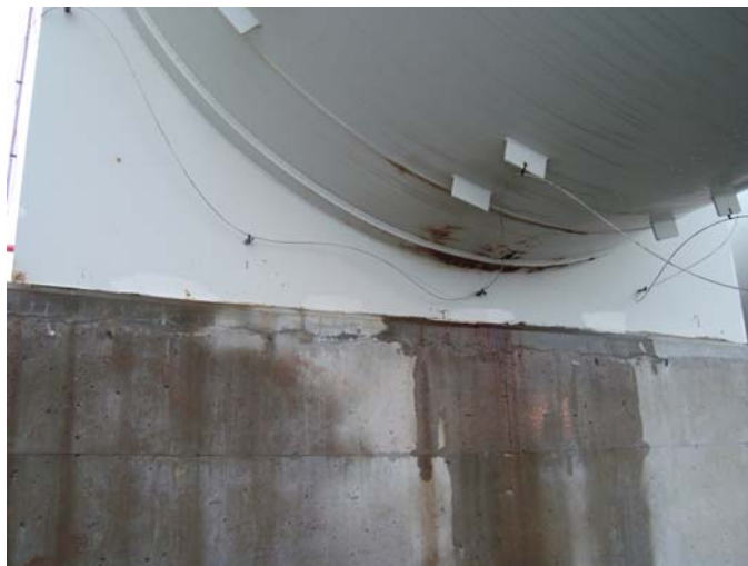
Photo 4 – South face of South vessel support showing coating breakdown on upper flange, photo taken facing North
