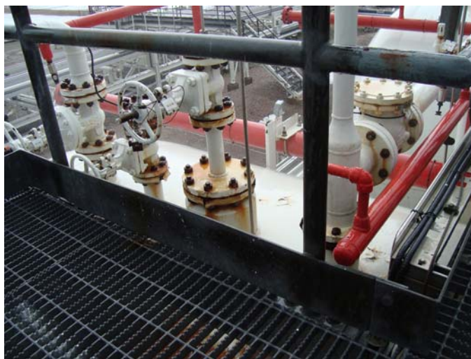
Photo 24 – Nozzles N3A, N4A, N8 & N1 showing coating breakdown, studs and nuts CAT III
