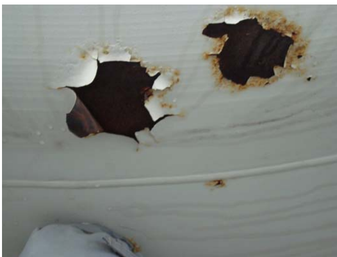
Photo 36 – Patches of coating breakdown, the largest measuring approx 160mm x 160mm under North end dome next to nozzle N10
