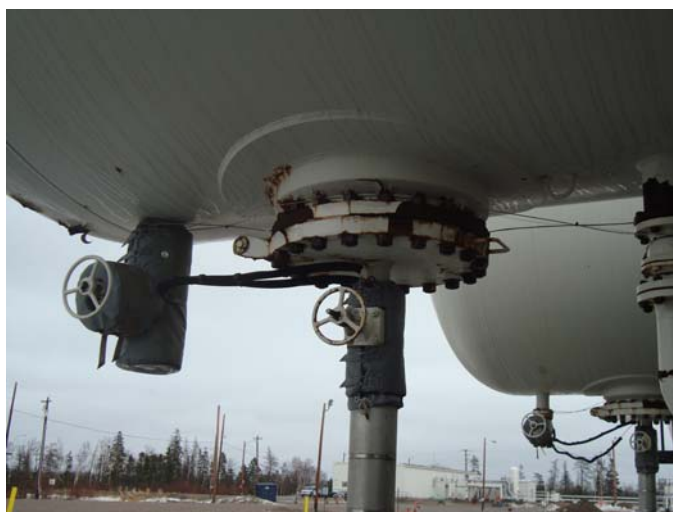
Photo 16 – Manhole with coating breakdown and light corrosion, studs and nuts CAT III
