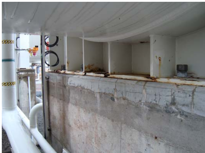
Photo 3 – South face of North vessel support , showing corrosion running along lower flange connection to concrete support, photo taken facing South
