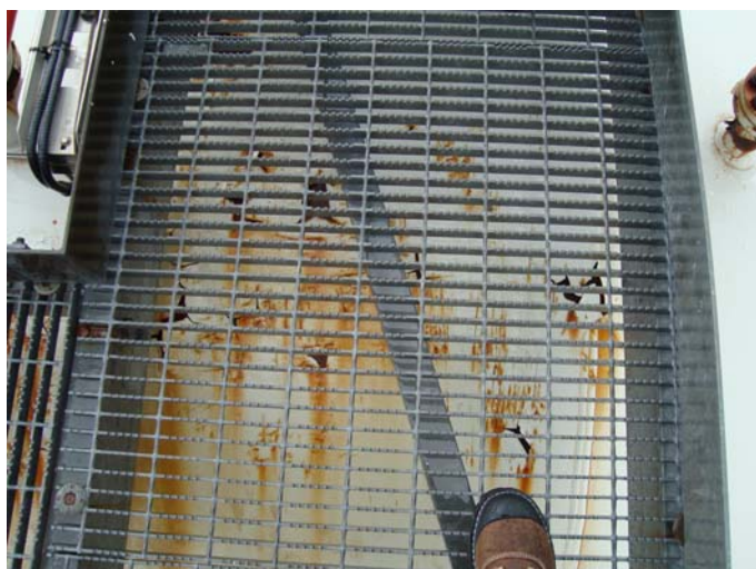
Photo 31 – Coating breakdown on top of vessel under South side walkway
