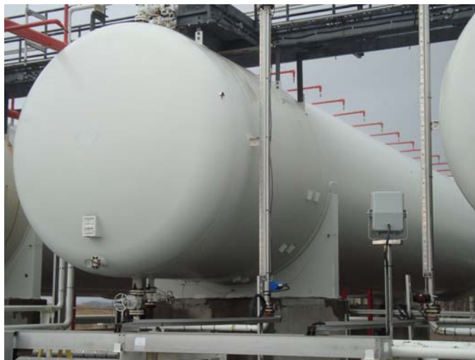
Photo 18 – General photo taken of the South end dome of vessel, showing one isolated patch of coating breakdown, photo taken facing North
