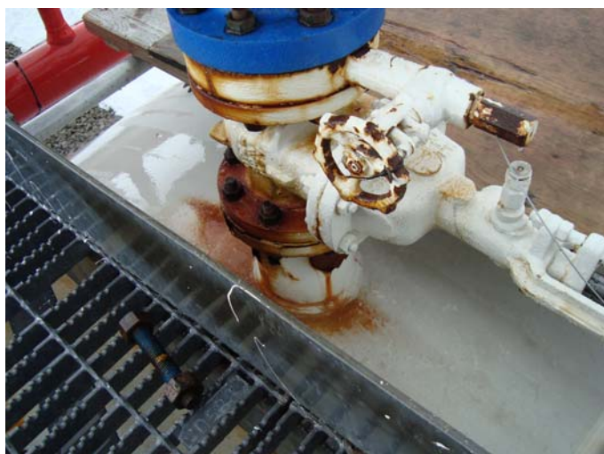
Photo 27 – Nozzle N7 with corrosion and coating breakdown
