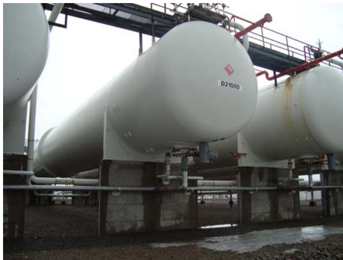
Photo 20 – General photos taken of North end dome of vessel, showing two isolated patches of coating breakdown on bottom centre of the dome end, photos taken facing South
