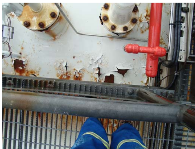
Photo 32 – Showing coating breakdown on top of South end dome next to nozzles N3A, N4A, N8 & N1
