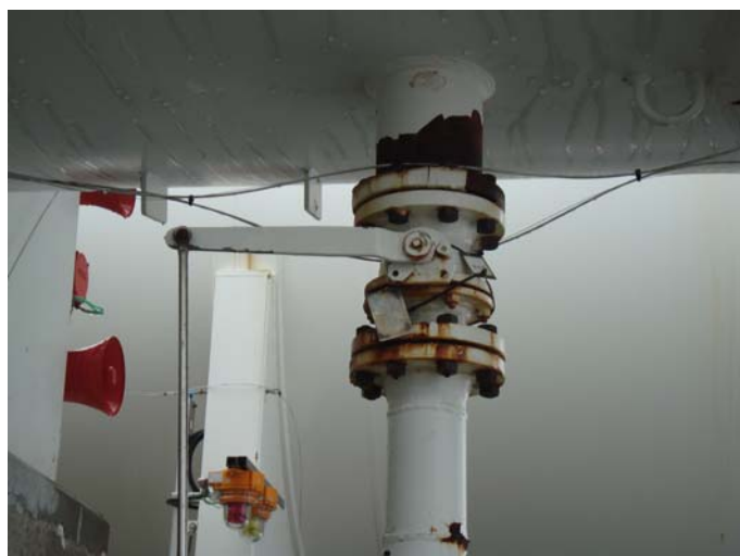
Photo 15 – Nozzle N5 with coating breakdown and light corrosion, studs and nuts CAT III
