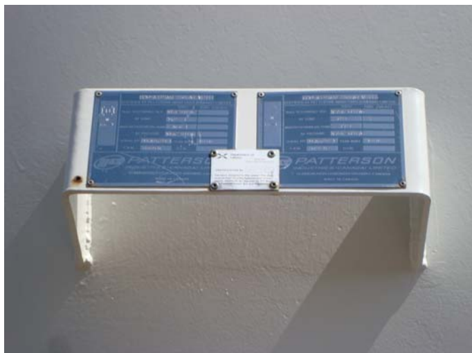
Photo 15 – Nameplate and Cal. Cert. No close visual, access platform deck 3.0m below plate.
