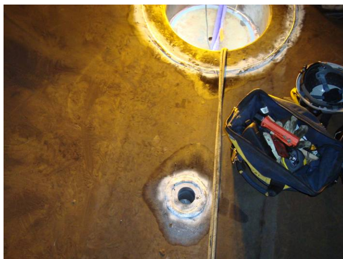
Photo 13 – Looking down at nozzle N5-3" from the interior at the North end
