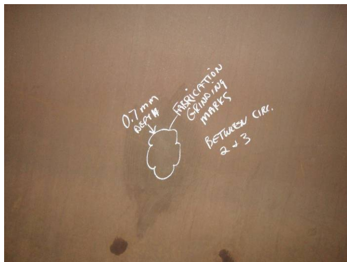
Photo 12 – Mechanical marks on interior shell surface between circ welds #2 and #3, looking East
