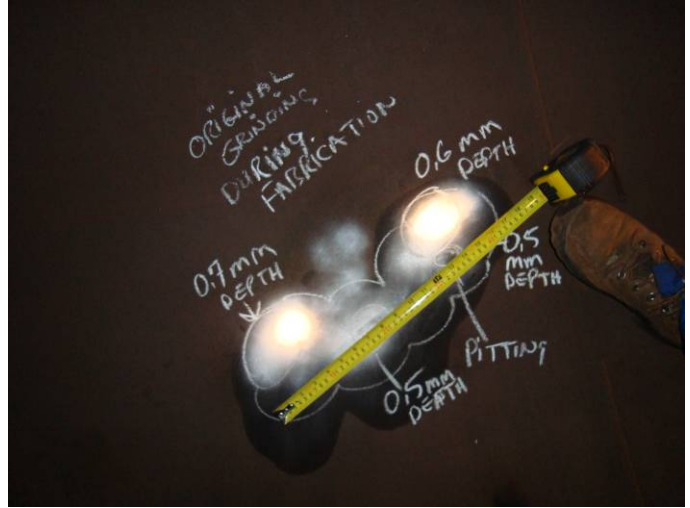
Photo 8 – Mechanical marks on localized corrosion pit looking West between #6 and #7 circ welds
