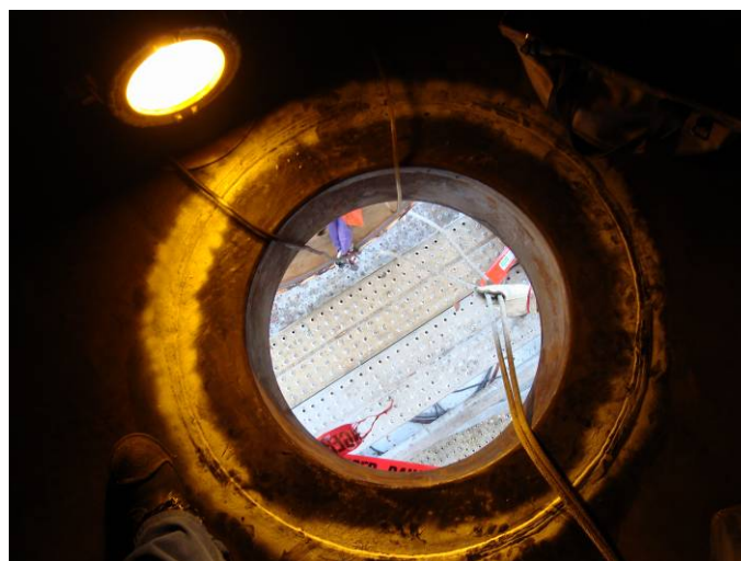
Photo 14 – Looking down at manway M-24" from interior of vessel at North end
