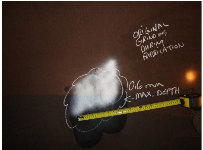
Photo 10 – Mechanical marks on interior shell between circ welds #3 and #4
