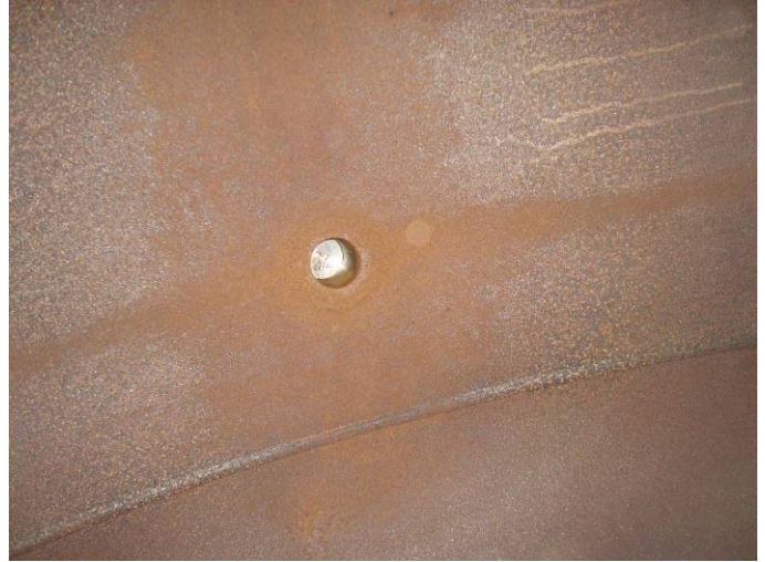
Photo 16 – Looking up at nozzle N7-4” from inside of vessel at North end
