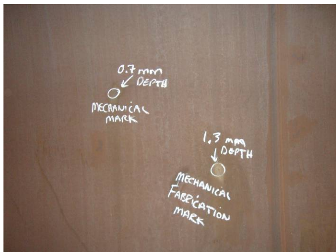
Photo 11 – Mechanical marks on interior shell just south of circ weld #3, looking West
