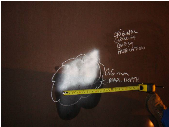
Photo 9 – Mechanical marks on interior shell between circ welds #3 and #4
