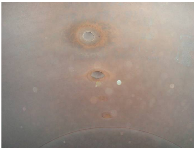
Photo 4 – Looking up at nozzles N3A-3”, N4A-2”, N8-6”, and N1-4” at South end of vessel interior
