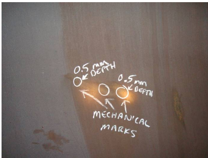
Photo 6 – Mechanical marks on shell looking West inside vessel between #8 and #9 circ welds
