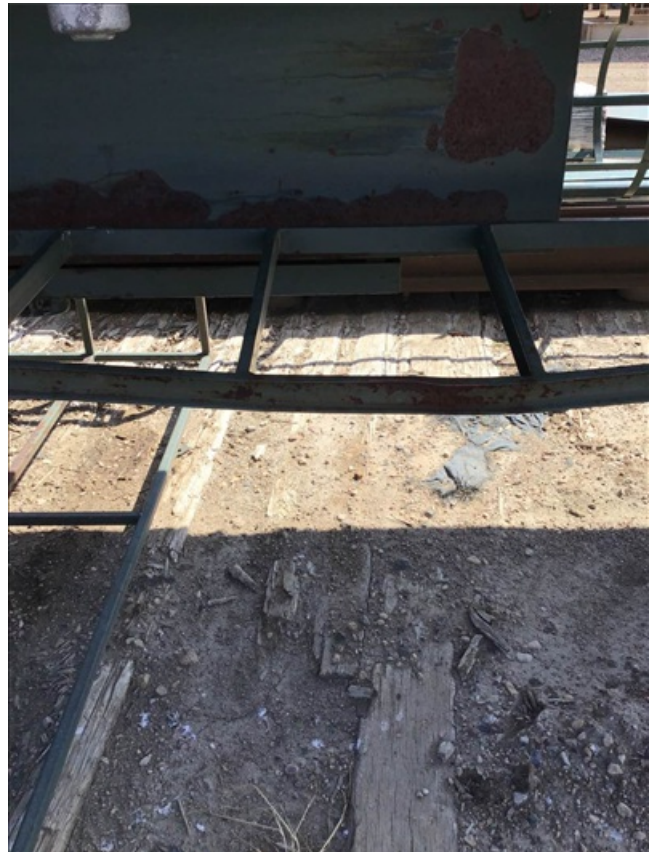
UPPER LADDER & CAGE
